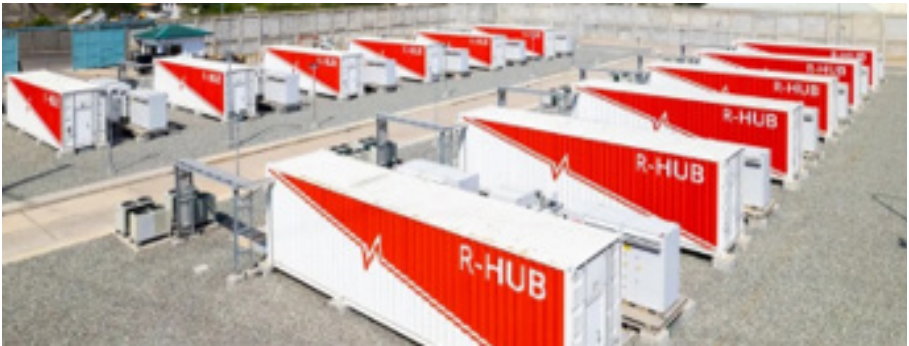
SMC has invested in battery storage facilities throughout the country to help ensure stable, reliable electricity while supporting the integration of more renewable capacities to the grid.
